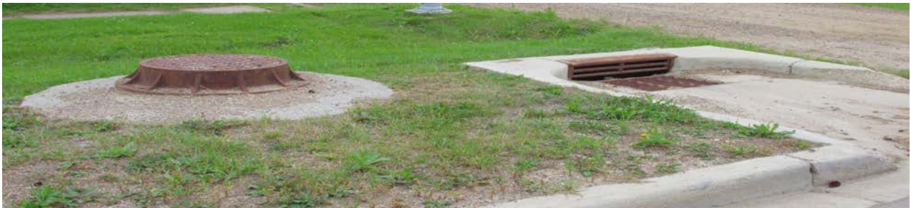
Catch basin and drainage man hole on south side of 100 Avenue, east of 100 Street
